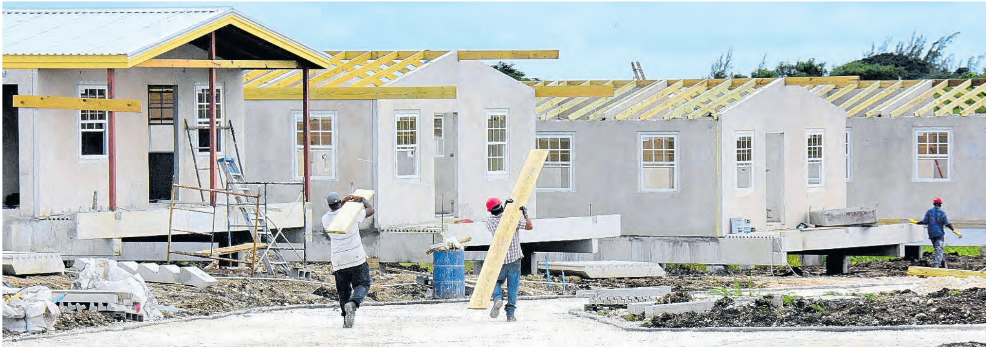
Workmen at Ridge Meadows, Christ Church, where more than 600 houses are being built.
