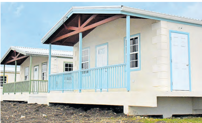
Some of the houses being built at Ridge Meadows, the Ridge, Christ Church. (Pictures by Reco Moore.)
